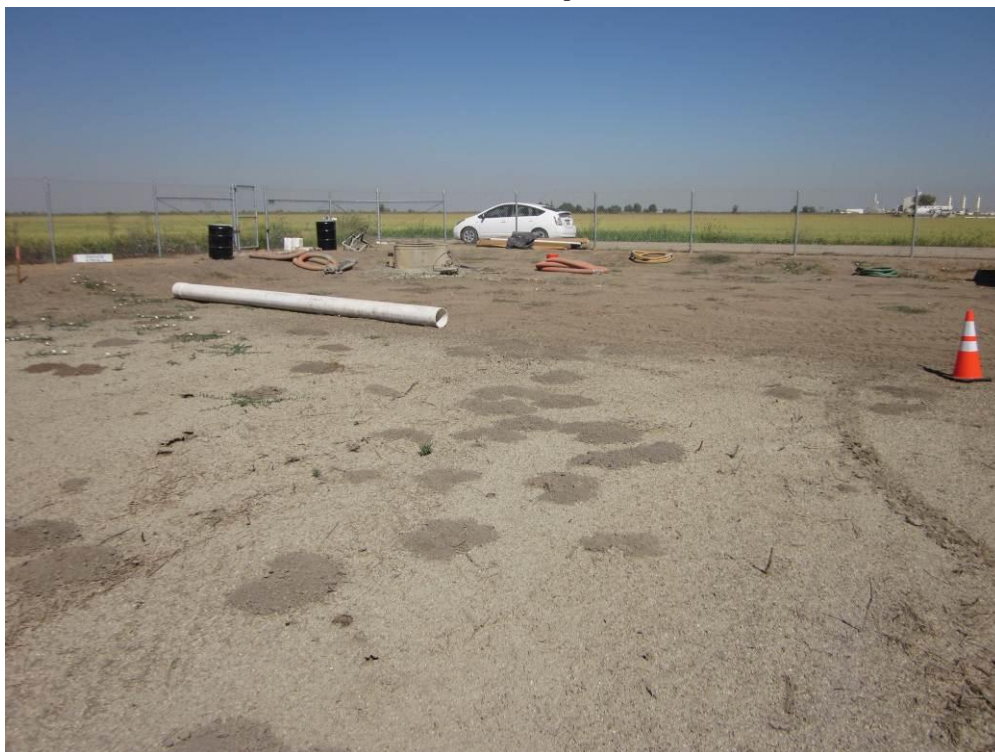
Photo 2: Drilling for the anode bed well in the northwest corner of the Remote Well Pad site has been started. The drill rig was being repaired at the time of inspection.
