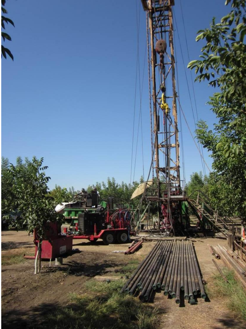
Photo 3: Well conversion activities have been initiated at the Southam #2 well site. The drill rig has been set up and drilling was actively underway. Pipe and equipment was observed outside the approved work area. This incident was reported to CVGS on September 13, 2012 and corrective action was taken and reported to the CPUC on September 14, 2012.
